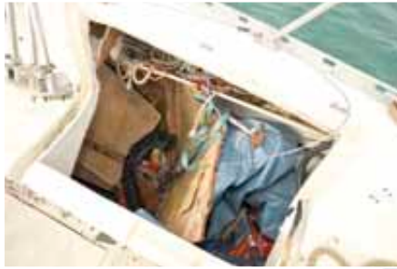
ABOVE: A bulkhead in the starboard cockpit locker was blown backwards by the blast
