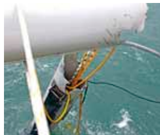
The egg-shaped holes for the lower coquilles proved to be a weak point. That's where it broke
